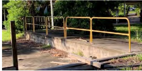
Fig. 4.9.4 Substandard Pedestrian Railing
