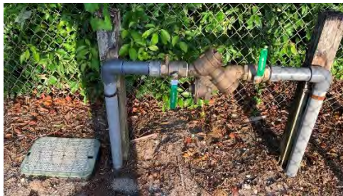
Fig. 4.9.8.B – Irrigation Backflow Preventer
