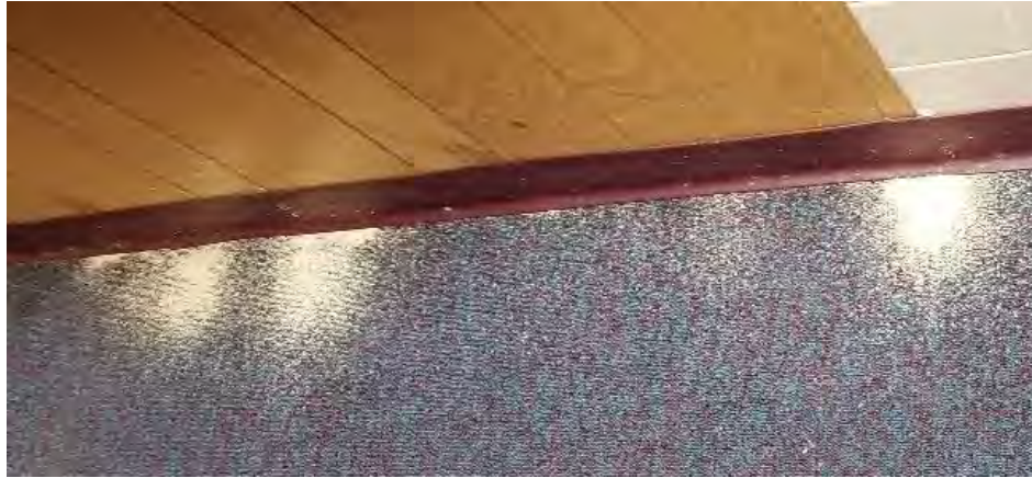
Fig. 4.10.3 Building 5 Potential insect damage
