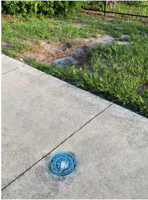
Fig. 4.9.8.A – Potable Water Meter & Fire Line Valve
