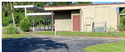
Fig. 4.9.3 Substandard Accessible Parking
