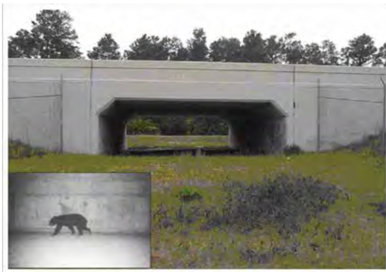
Prefabricated concrete box culvert along SR 46 in Seminole County, Florida. (Source: Wildlife Crossing Handbook Randy S. Kautz, Stephen R. Bittner, and Tom H. Logan)
