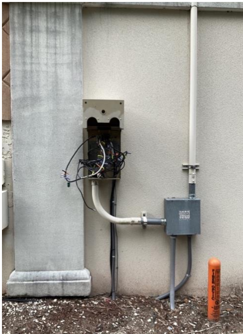
Figure 13 – Open and Exposed Spectrum Service Drops St John Parkway
