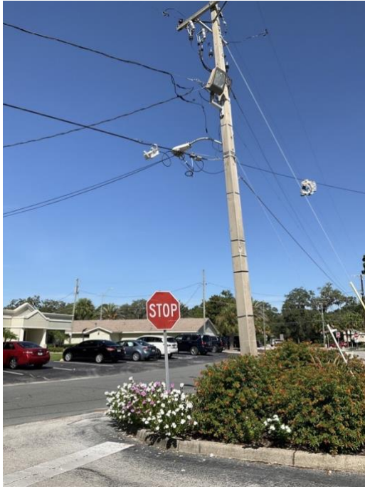
Figure 11 - Spectrum WI-FI AP Broken Strand Hanger Piney Ridge Rd
