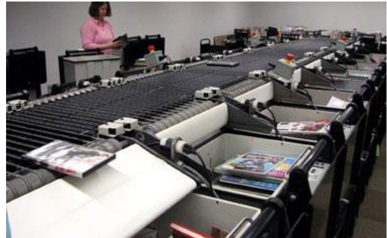
Automated materials handling system sorting books into bins, circa 2010, enabled by RFID tags in each collection item for better inventory control, as well as rapid, more accurate sorting to get items back on shelves faster, Champaign Public Library, Champaign, Illinois
